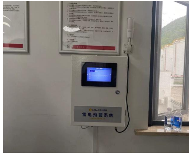
Early warning main box
